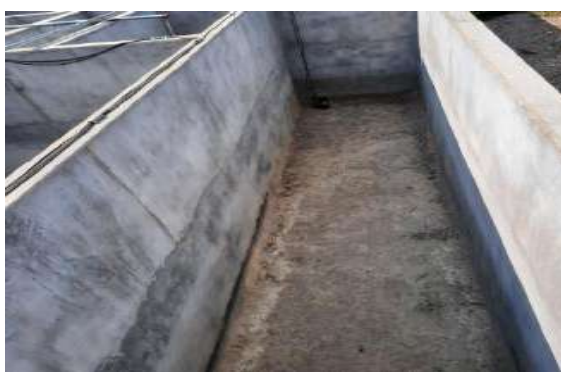
Bể trung gian
